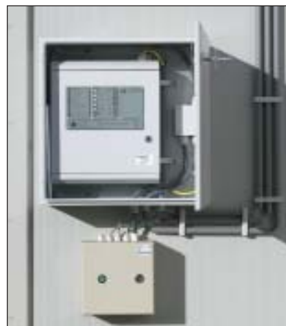
Fire detection system
